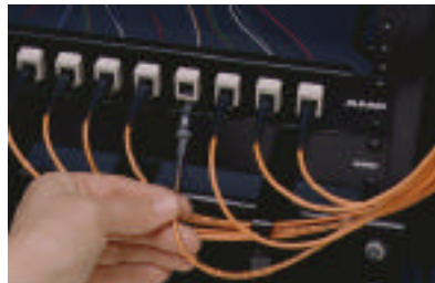
MT-RJ at the patch panel
