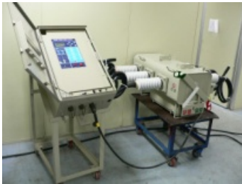
CB & Switch with sensors
