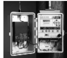
Capacitor bank control
