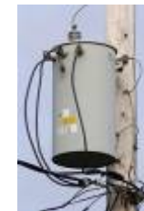
Pole mounted Transformer
