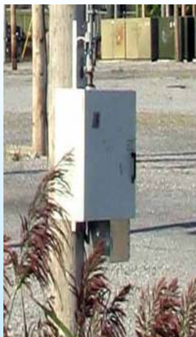
Standard control cabinet
