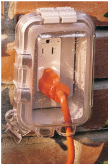
Figure 22 In-Use Weatherproof Receptacle Cover
