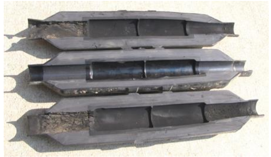
The center splice body is a non-faulted splice from the same location on different phase, this splice is in good condition.
