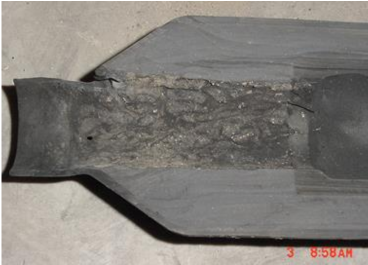
Close-up view of erosion of splice body
