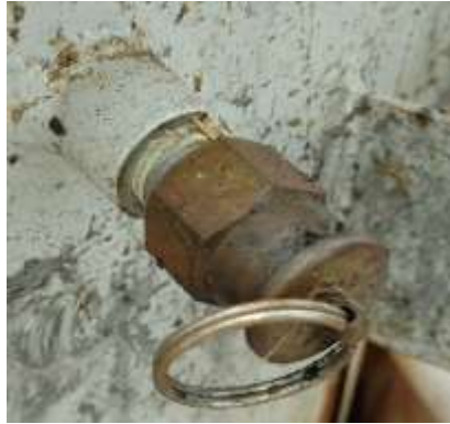
Figure 12: Silicon-Bronze Pressure Relief Valve on Stainless Flange (Welded to Steel Tank)
