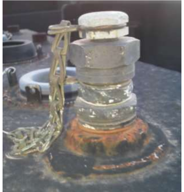
Figure 7: Bronze Sampler Valve on Steel Pipe Flange
