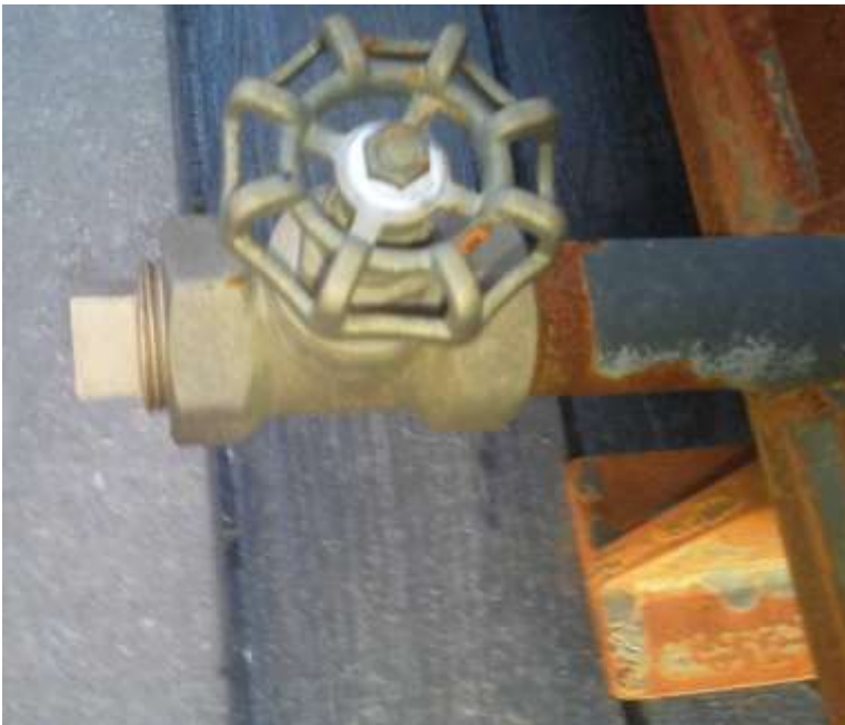
Figure 8: Bronze Drain Valve on Steel Pipe
